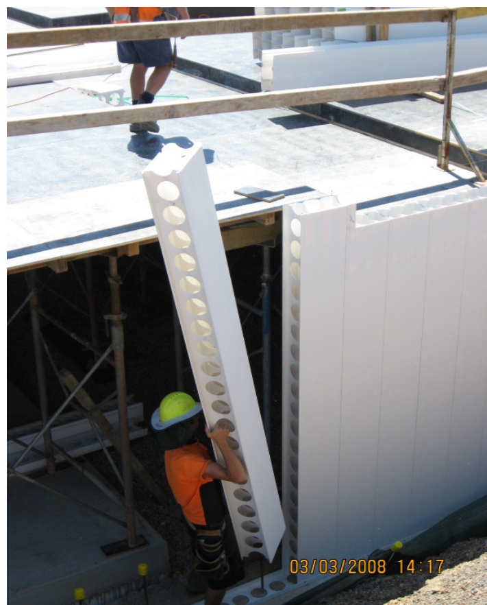
Photo courtesy of AW Edwards installing Dincel Construction System at Norwest Private Hospital
